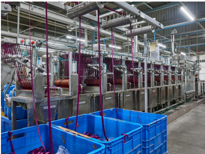
Tape Dyeing facility at Hassan, Karnataka
